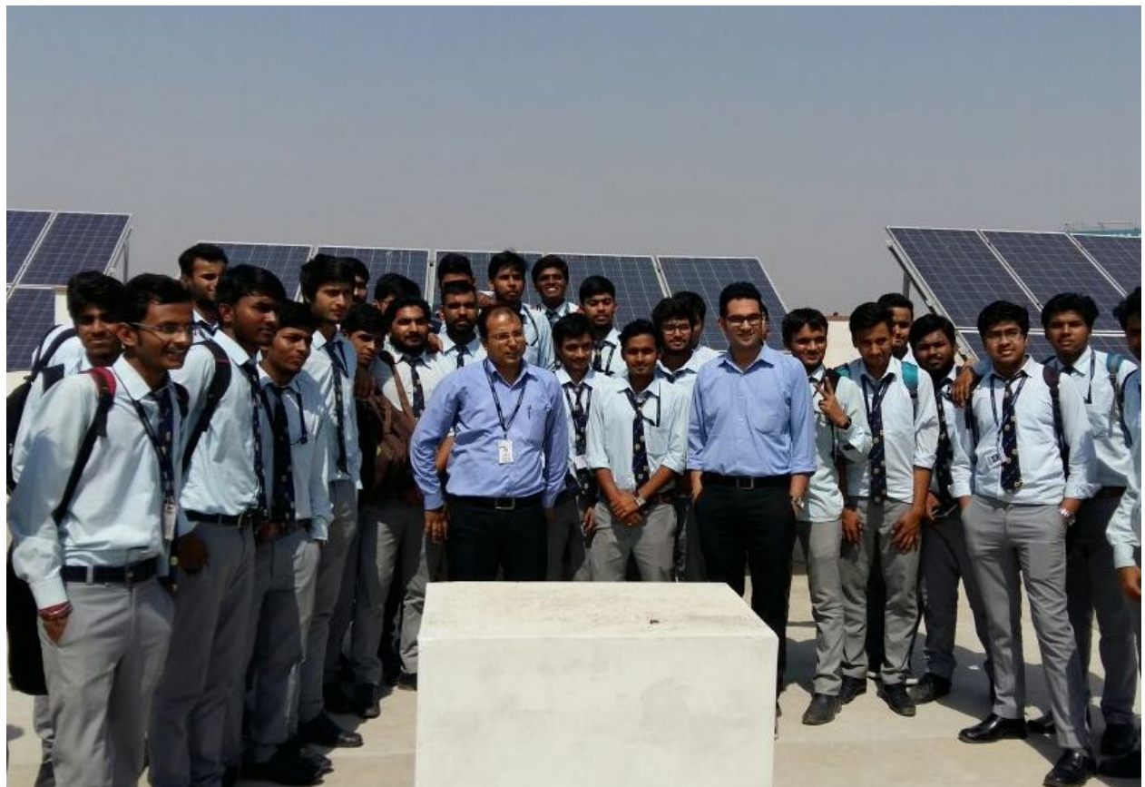
100 KW Solar Power Plant Visit of PGI Mechanical Students at Poornima University
